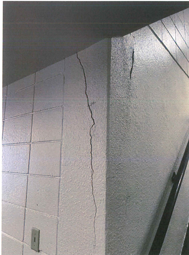
Photo-1: Damaged beam bearing at second floor level.
