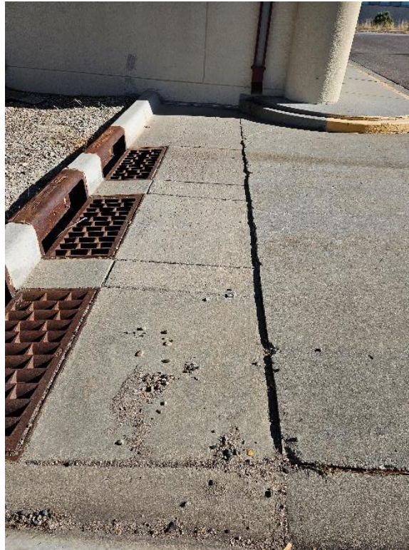
Photo 6: Drainage challenges at Business Building
