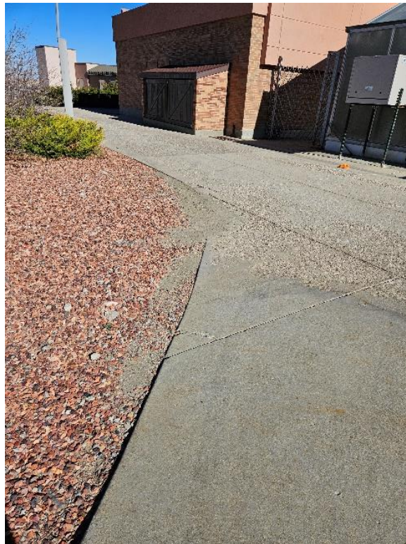
Photo 3: Evidence of sediment accumulation and ponding water
