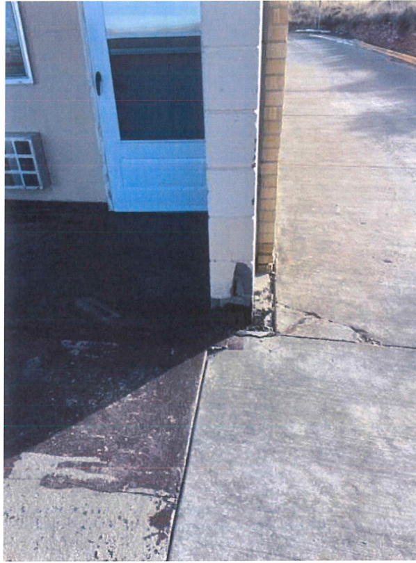
Photo-4: Damaged CMU at south-west corner. This damage should be repaired with an epoxy Mortar patch.
