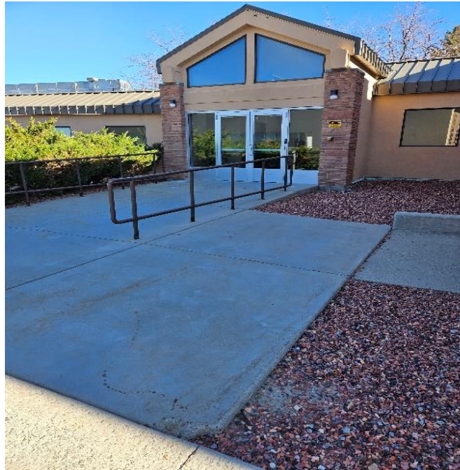
Photo 4: Poor drainage near west entrance to Loftin Life Science Building and Aley Hall
