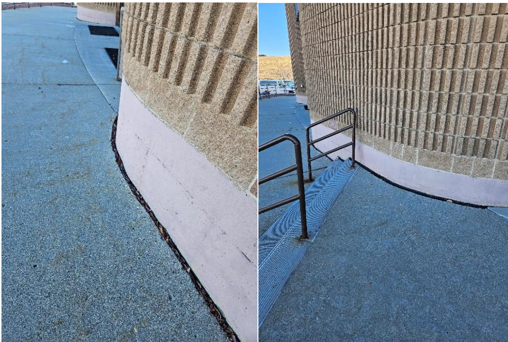
Photo 8: Concrete settlement along north face of Krampert Theater
