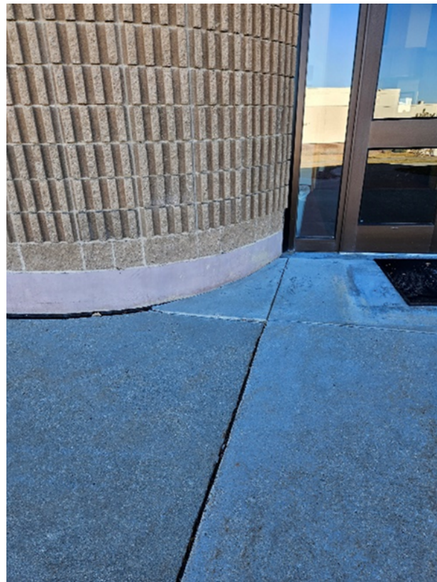
Photo 10: Pavement movement at the north side of Krampert Theater
