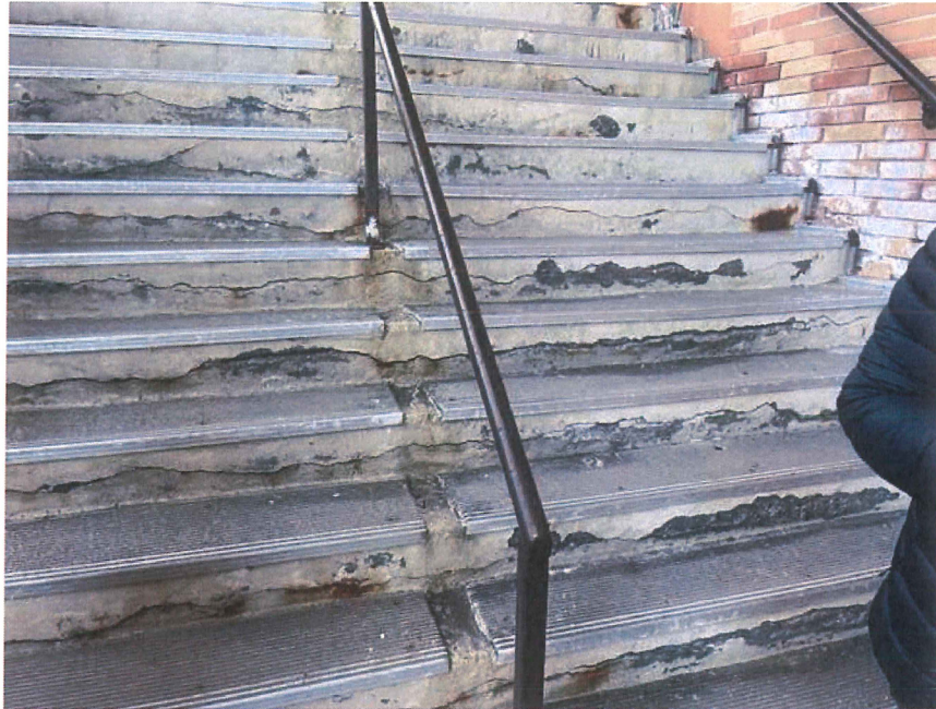
Photo-2: Damaged exterior stairway at north-east.
