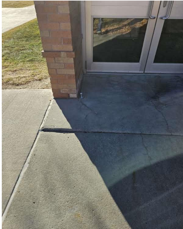
Photo 9: Pavement movement at the Saunder's Health Science west entrance
