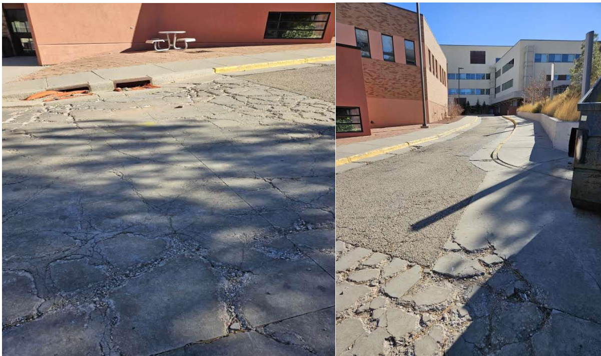
Photo 1: Poor drainage between Physical Science and Business Building
