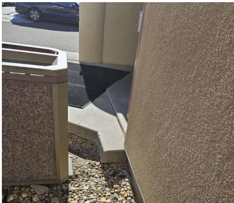
Photo 12: Pavement movement at the Business Building south door
