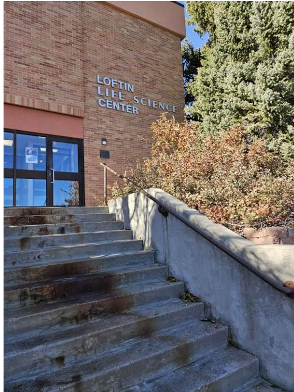
Photo 15: No direct ADA entrance to Loftin Life Science Building
