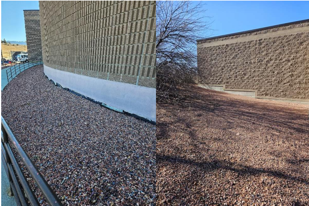
Photo 7: Inadequate landscaping and cover around the Krampert Theater
