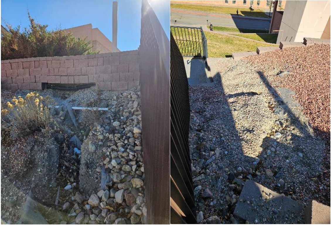
Photo 2: Damage downstream of Physical Science and Business Building
