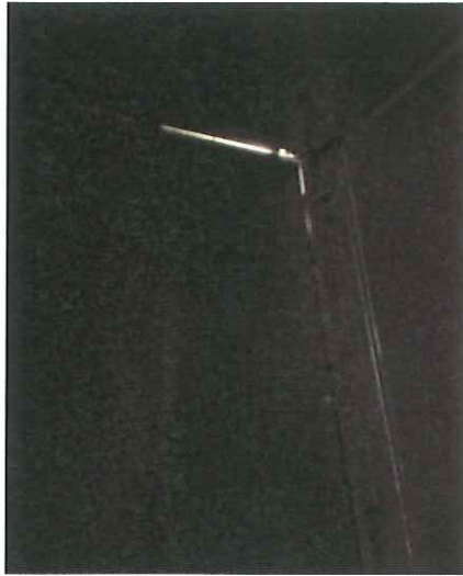
P3.2 & 3.3: Supply Discharge Compartment - Gap in Corner of Section A Wall
