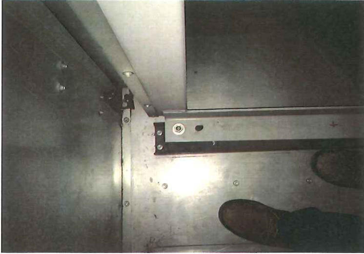
P4.1: Supply Fan #3 - Isolator Rail Reinstalled with Fan Off Square to Inlet Block-Off Wall
