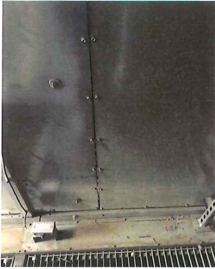
P3.1: Supply Discharge Compartment - Gap in Section A Wall
