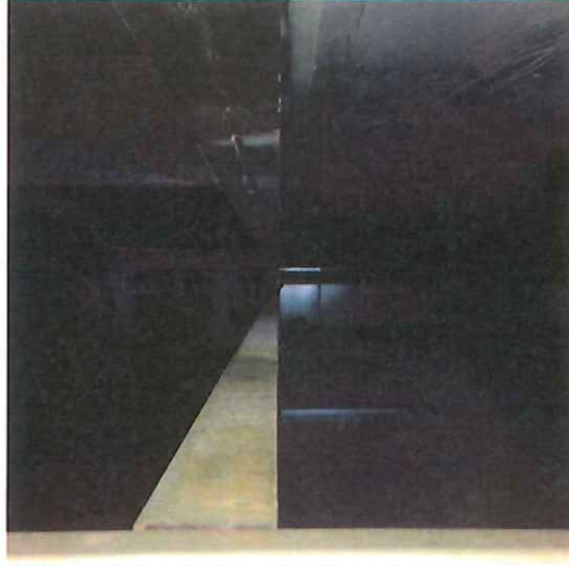
P2.2: Section Splits Under Unit Section C & D within Curb [No Spring or Curb Support to Slab]
