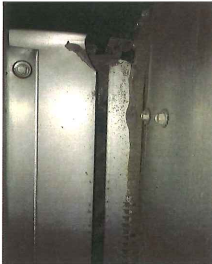
P4.3: Supply Fan #3 Inlet Flex Connection - Right - 1/8" Gap
