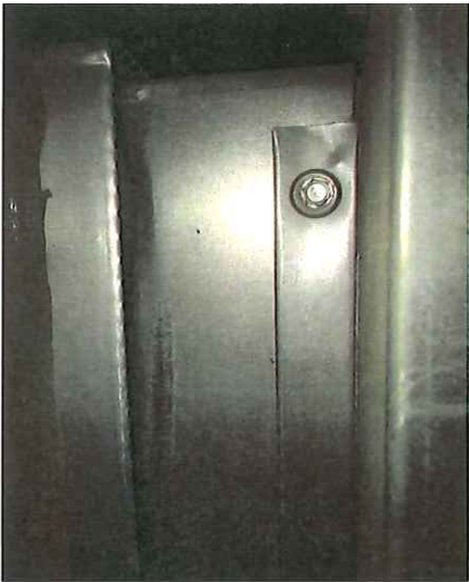
P4.2: Supply Fan #3 Inlet Flex Connection - Left - Impinged
