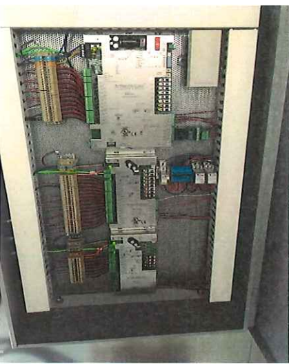
P1.4: Automated Logic Control Panel within Exhaust Section of Unit
