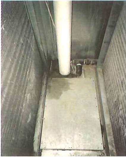
P2.6: HWC Piping Run Through Unit Flooring, Not into Pipe Chase
