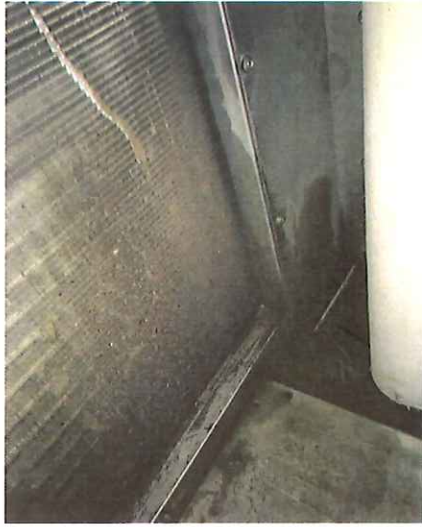
P2.7: Lower Right Corner of DX Cooling Coil - Potential Leak
